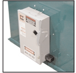
NEMA 3R service rated, fused main disconnect with lightning surge protection to safeguard station electronic components from power surge.
