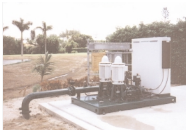
Little Club Delray Beach, FL 600 GPM VFD/EBV Pressure Regulation
