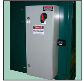
NEMA 4 service rated, main disconnect with lightning surge protection to safeguard station electronic components from power surge.
